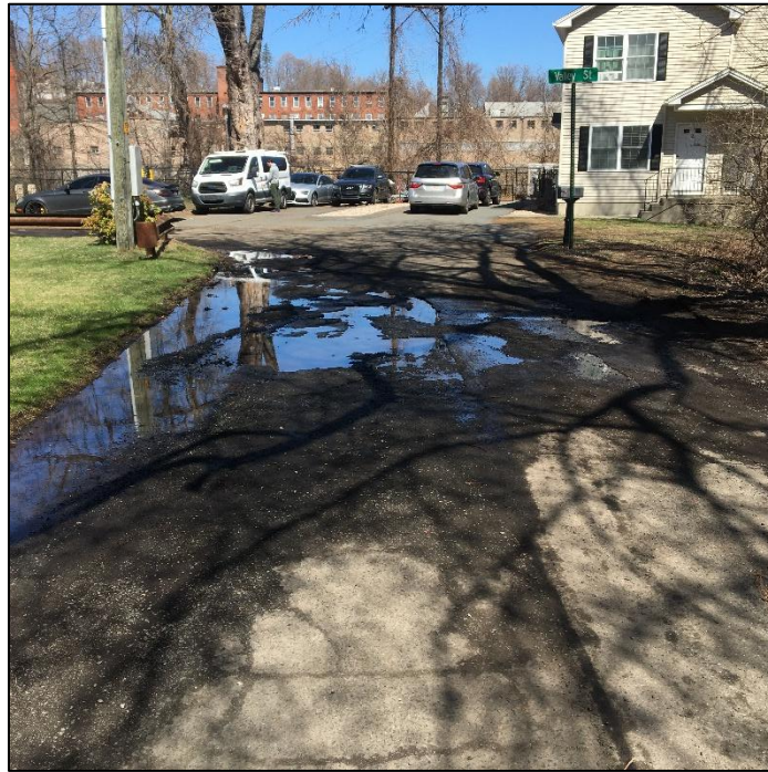
Photo No. 3. View of standing storm water at the northernmost portion of Moore Street. The location is within the 200-ft Riverfront Area.
