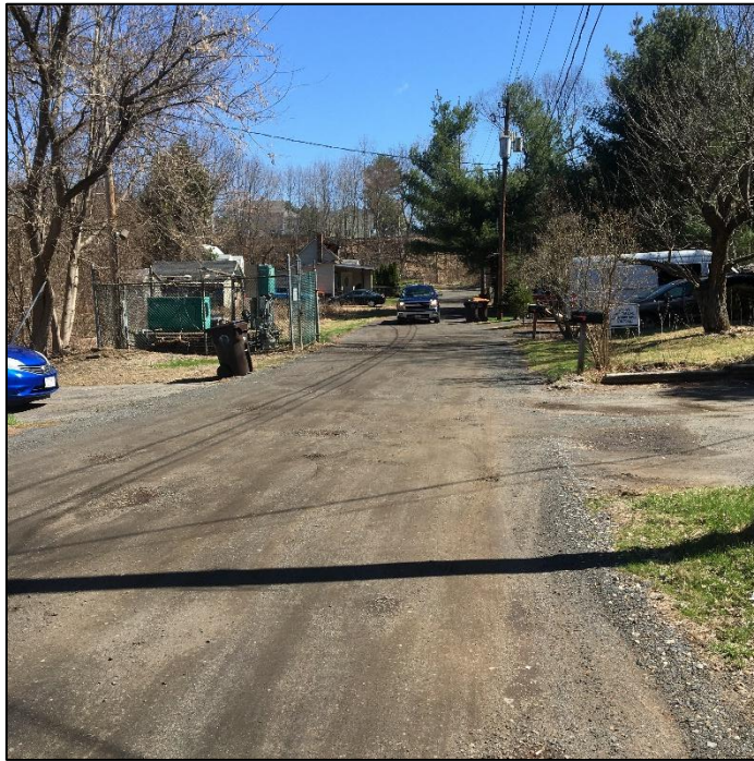
Photo No. 5. Typical pothole and undulating gravel surface condition on Valley Street (east).
