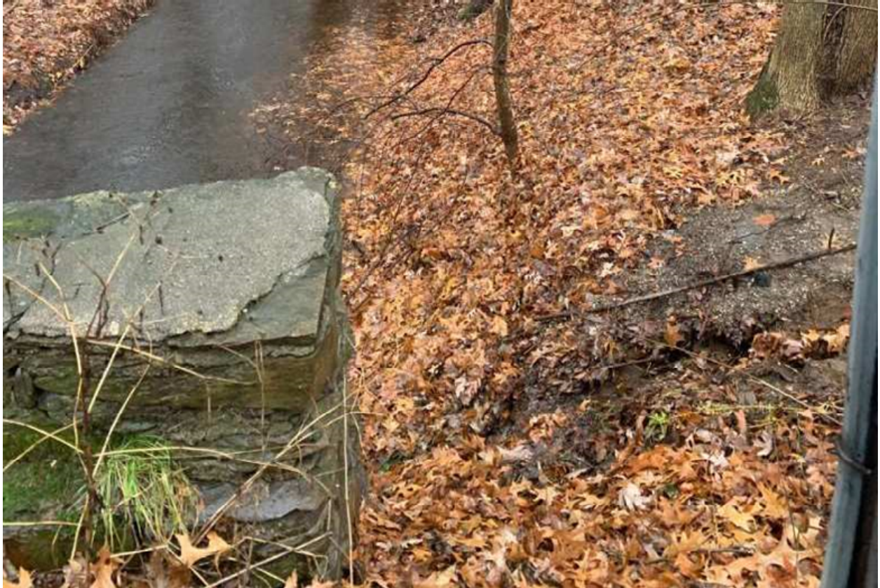
South West Street stream crossing, Erosion at end of paved swale – December 1, 2020
