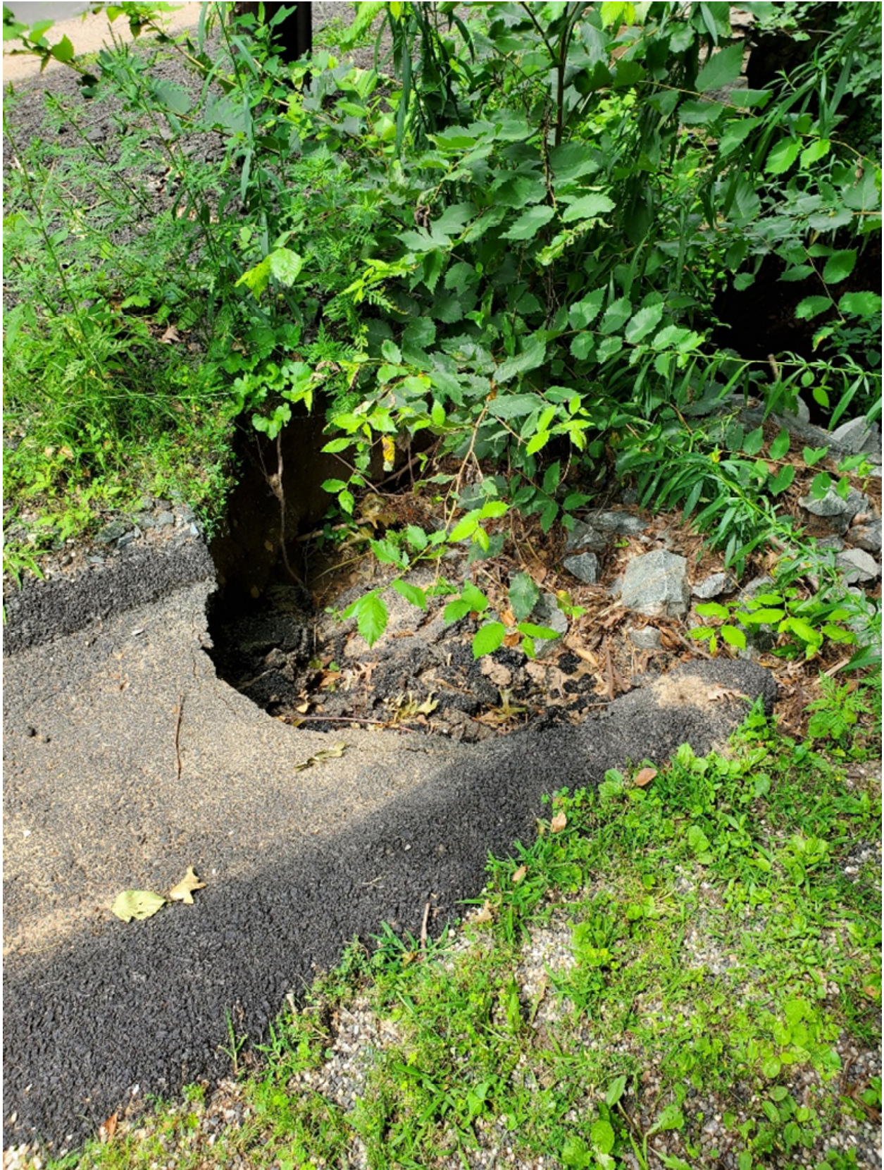
South West Street stream crossing, Collapse of paved swale at due to erosion by stormwater runoff – August 4, 2021
