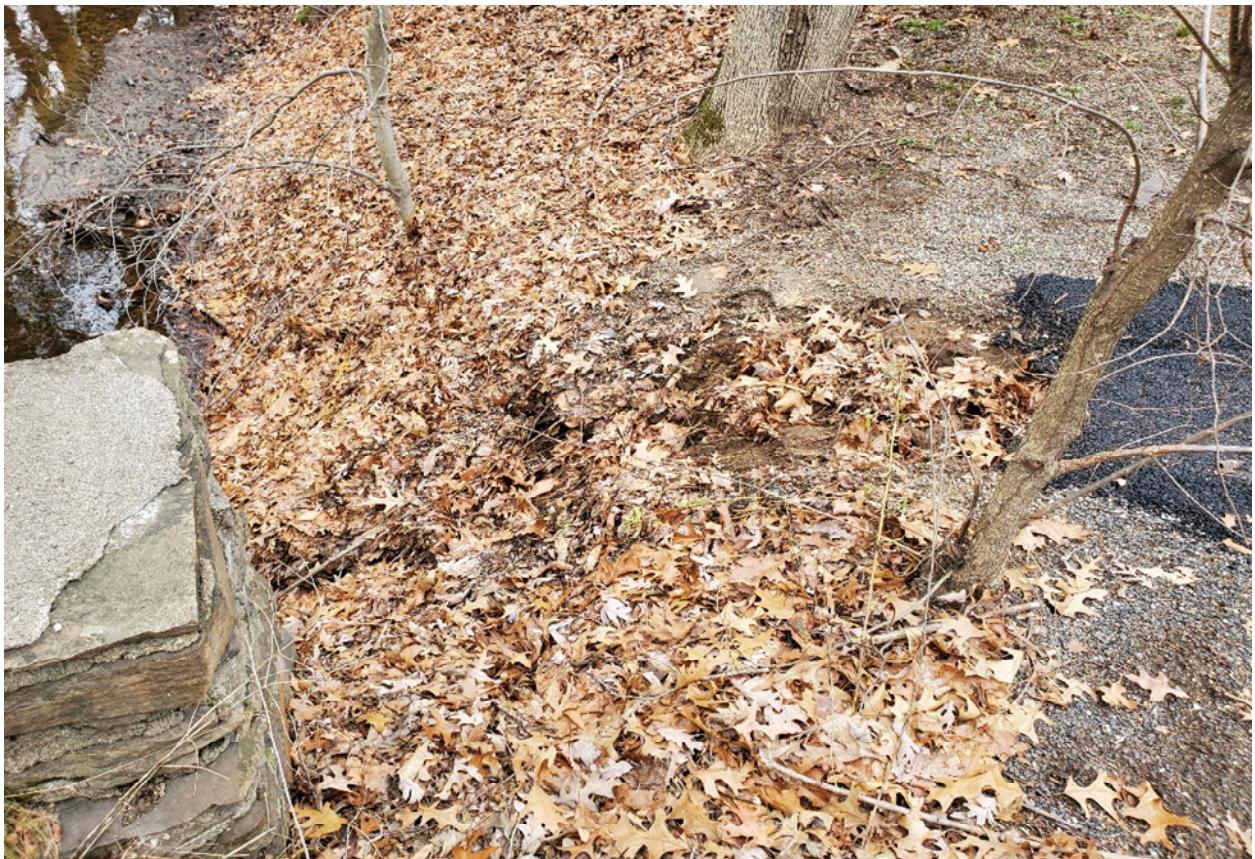
South West Street stream crossing, Erosion at end of paved swale – December 3, 2020
