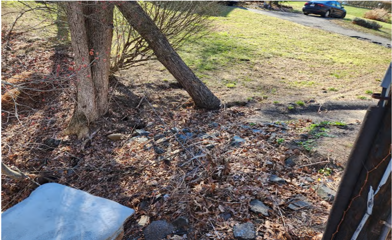
South West Street stream crossing, Tree damaged due to erosion – April 17, 2025
