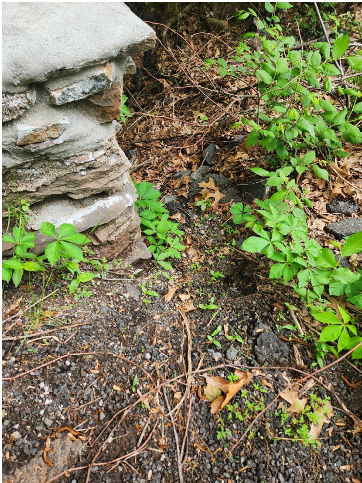
South West Street stream crossing, Erosion due to stormwater runoff along culvert headwall – May 16, 2025
