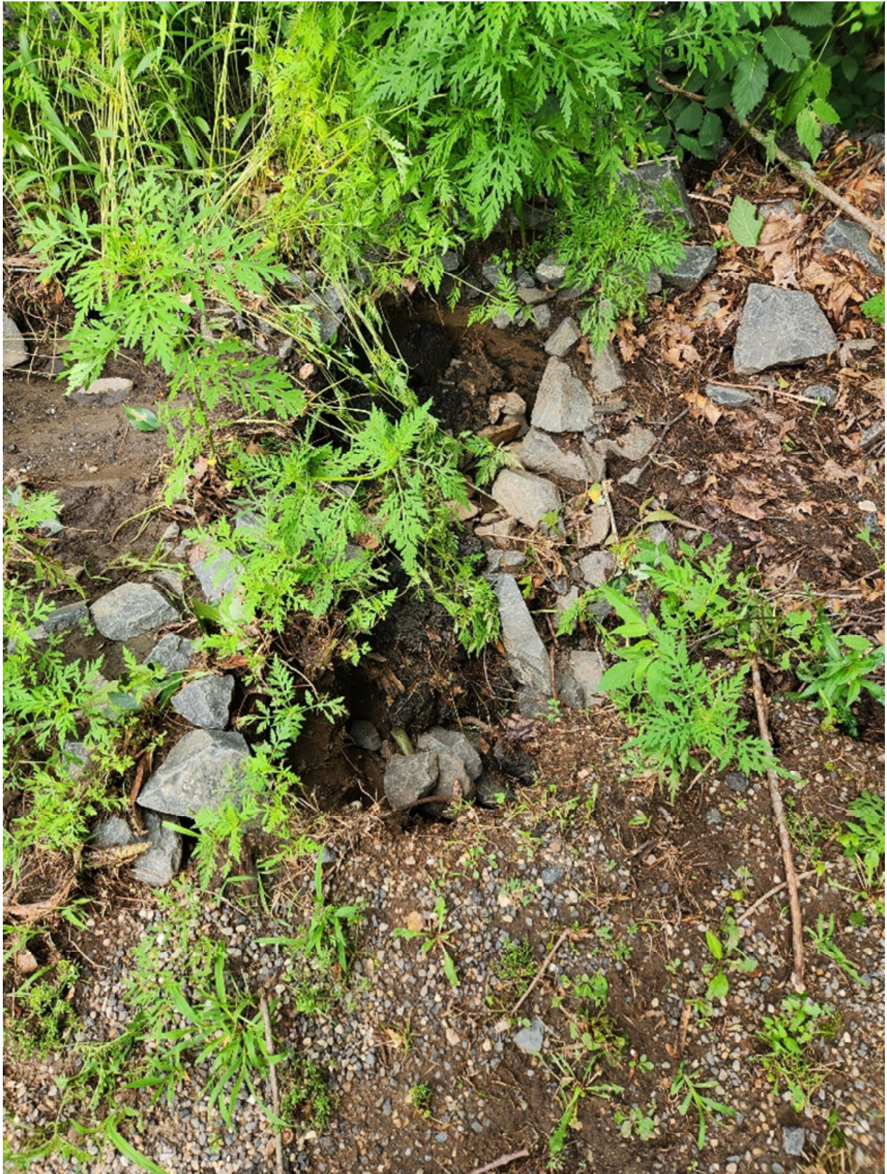
South West Street stream crossing, Erosion continues along edges of riprap area – July 19, 2023
