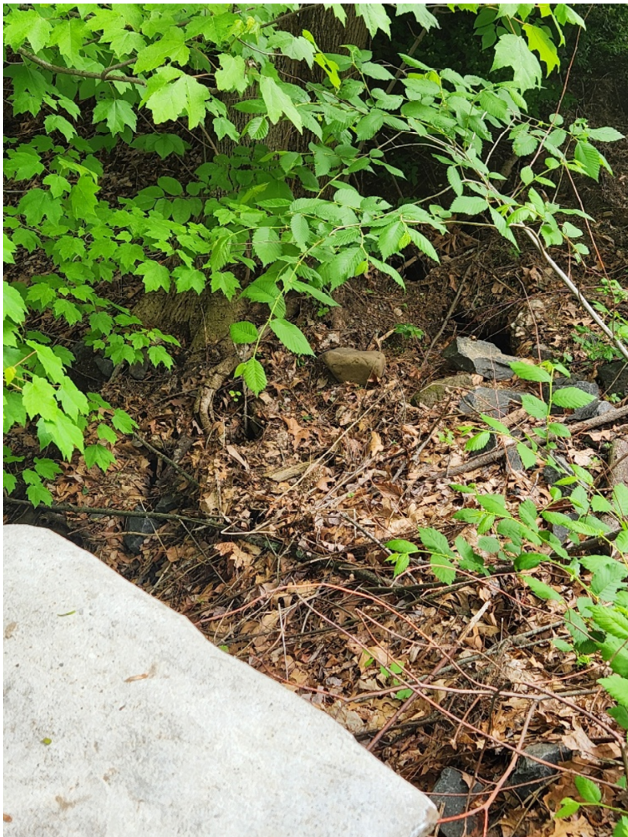
South West Street stream crossing, Continued erosion from runoff observed at stream bank – May 16, 2025
