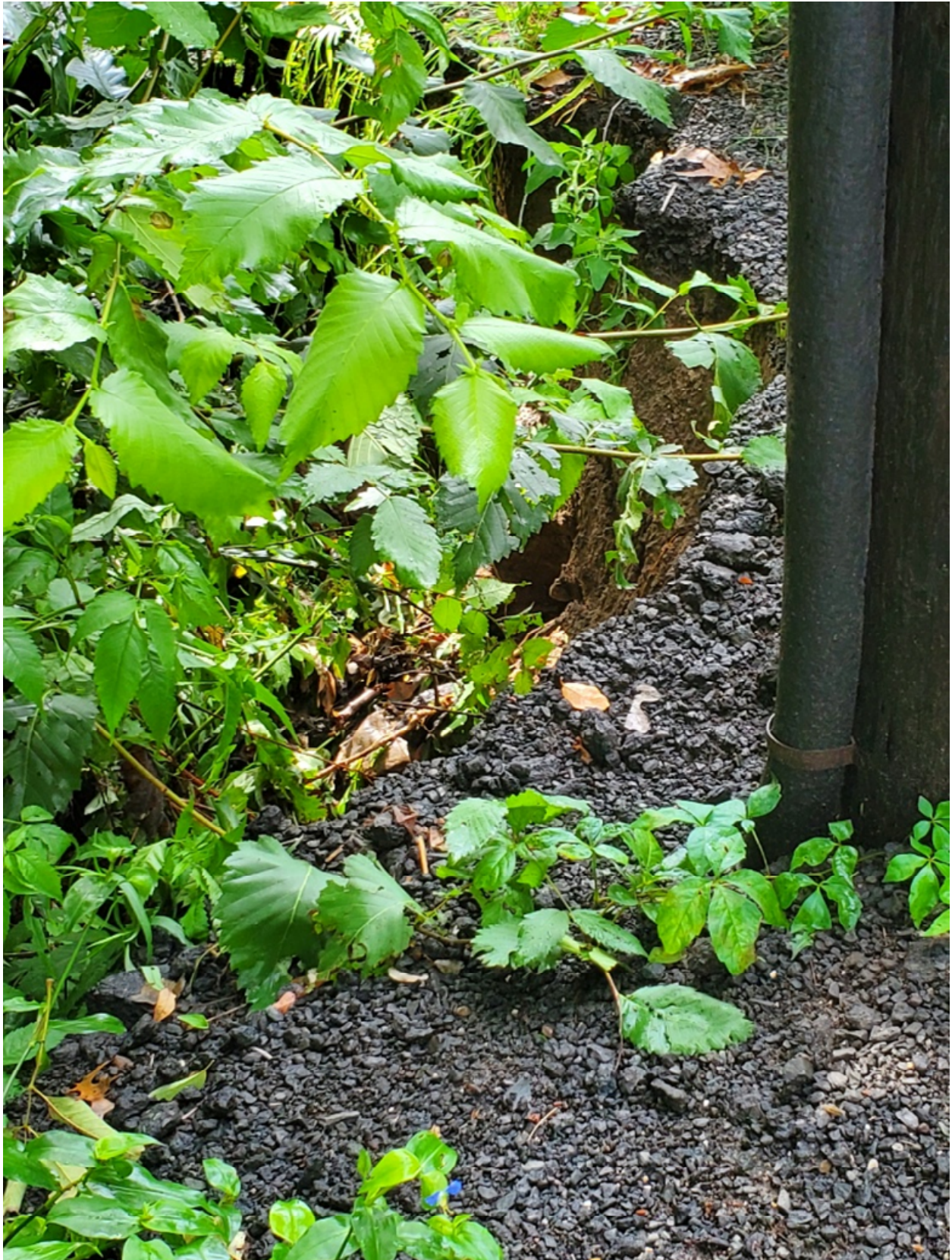
South West Street stream crossing, Erosion caused by stormwater runoff near utility pole – August 19, 2021
