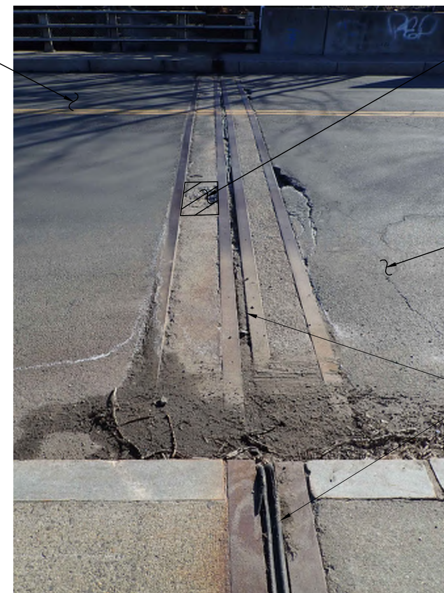
SOUTH ABUTMENT BRIDGE JOINT LOOKING EAST
