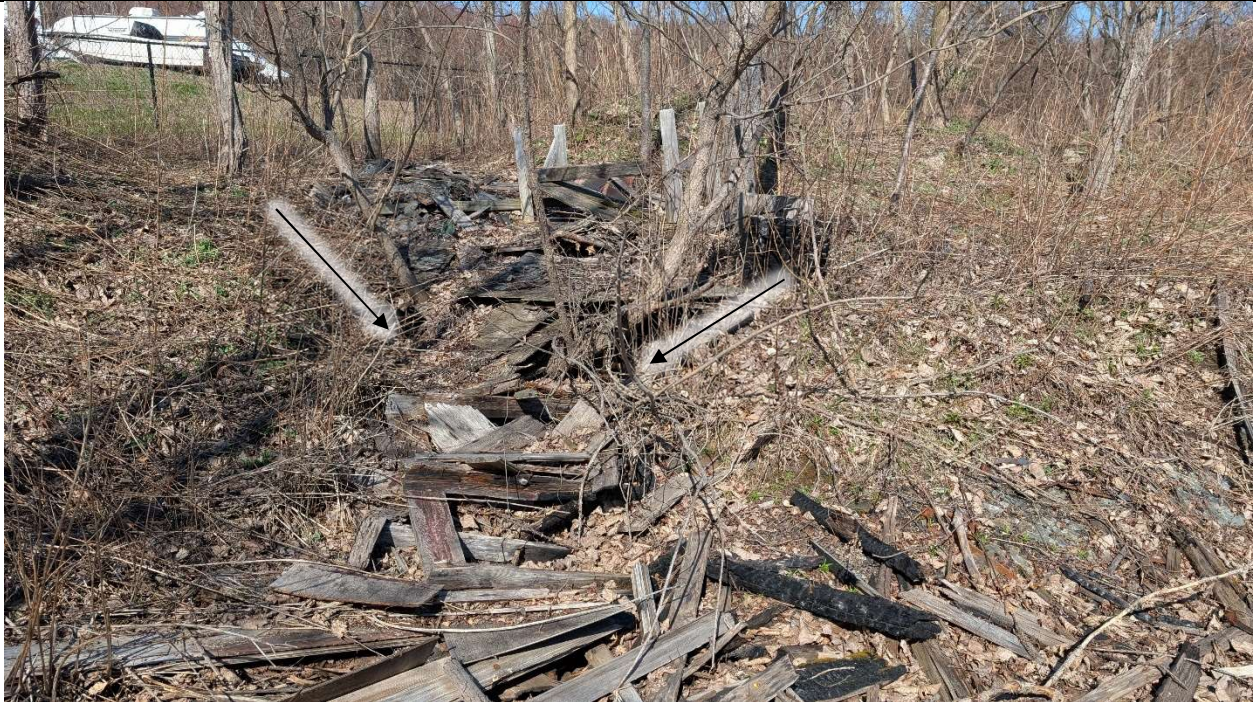
Figure 3. Closer view of the woody debris that is clogging the entrance of the trench. Arrows point to the entrance of the trench. Facing northeast.
